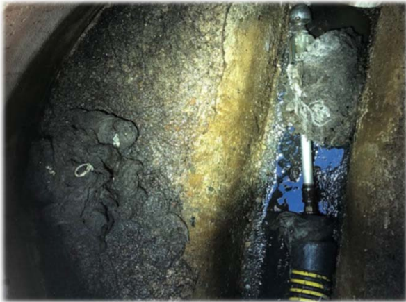
Partial Blockage Found During PM's
