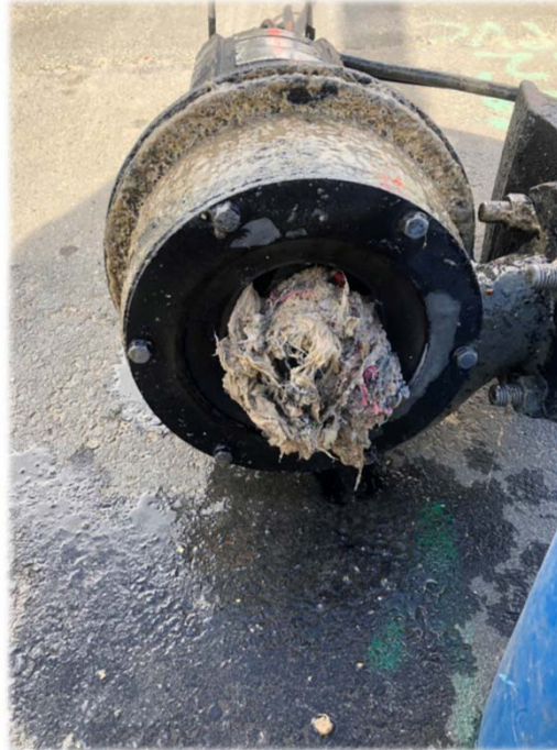
Clogged Chopper Pump
