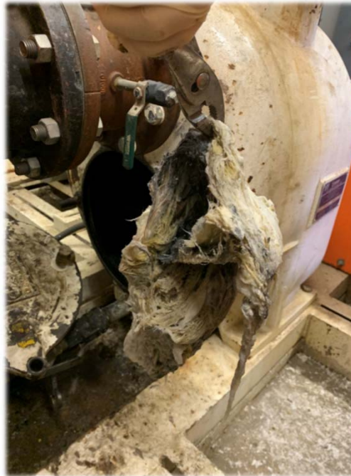
Clogged Centrifugal Pump
