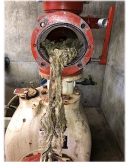
Clogged Check Valve
