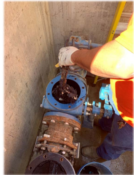
Clogged Check Valve
