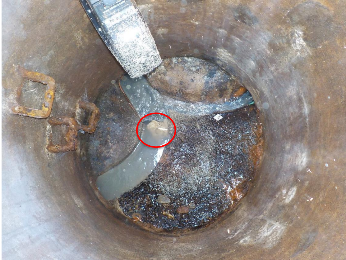
Confirmed channel grease obstruction dislodged upstream
